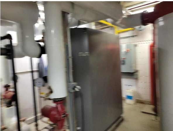
Photograph No. 43 Heating boilers are new and in good condition.
