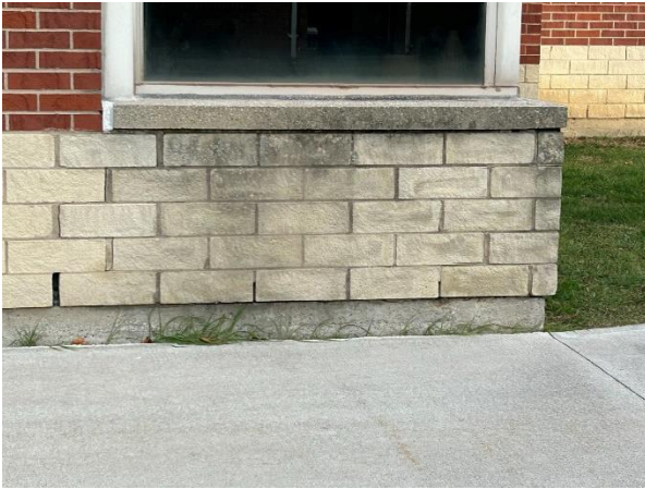
Photograph No. 5 Stone deterioration and staining below lower-level windows.
