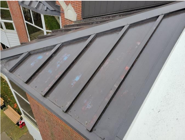
Photograph No. 19 Discolouration at sloped metal roofing.
