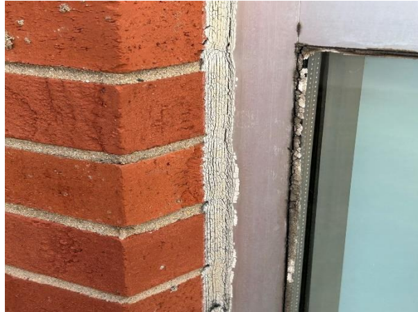
Photograph No. 10 Aged Sealant around windows
