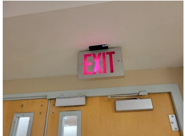
Photograph No. 56 Exit lights are in fair condition.
