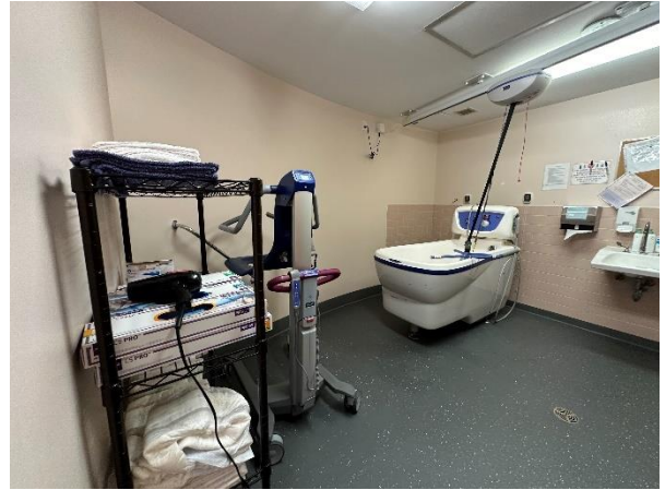
Photograph No. 30 Typical shower and tub room finishes are in good to fair condition.
