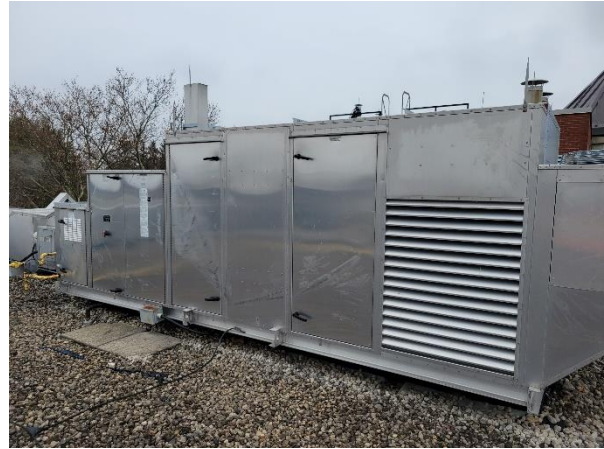
Photograph No. 46 All air handling units are new and in good condition.
