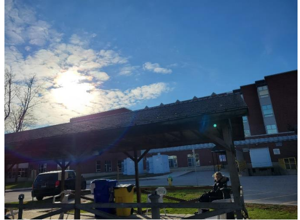
Photograph No. 70 The staff outdoor gazebo is in fair condition with the shingles being in poor condition.
