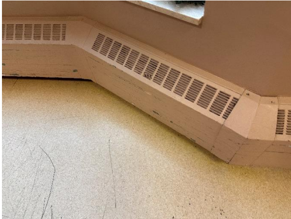
Photograph No. 37 Scratched flooring and radiators.
