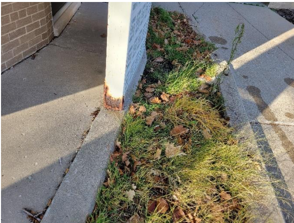
Photograph No. 11 Corroded metal framing at decorative screens.
