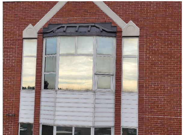
Photograph No. 8 Failed window film at the bay windows.
