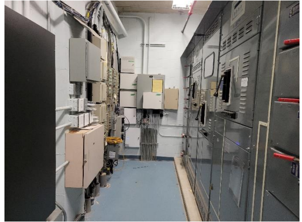
Photograph No. 54 Main electrical distribution equipment is in good condition.
