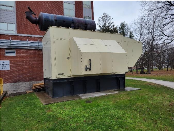
Photograph No. 51 Diesel generator appears to be in good condition with no issues reported.
