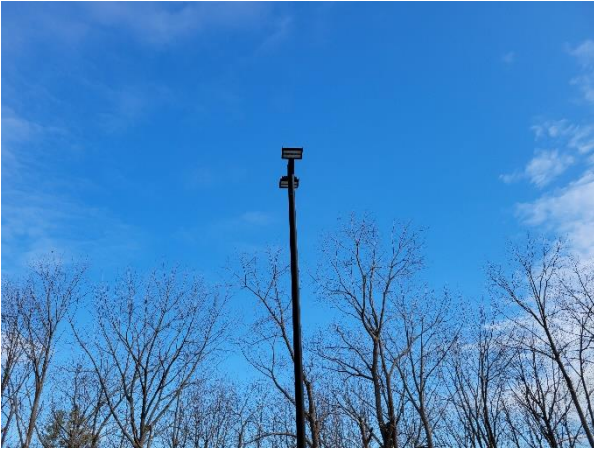
Photograph No. 61 Lamp standards with new LED lamps are in good condition.
