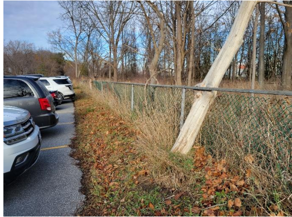
Photograph No. 62 Perimeter chainlink fence is in fair condition with damages noted.
