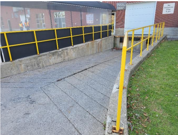
Photograph No. 63 The loading dock ramp is in good condition with localized concrete damage noted.
