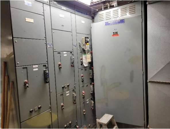
Photograph No. 53 Open electrical panel noted in MPH.
