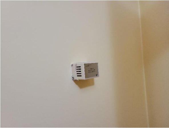
Photograph No. 57 Thermostats are pneumatic but reportedly operational.
