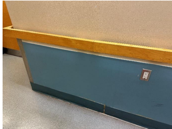
Photograph No. 24 Faded wood handrails.
