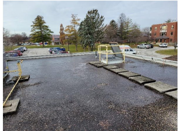
Photograph No. 16 Ponding water along south roof areas.
