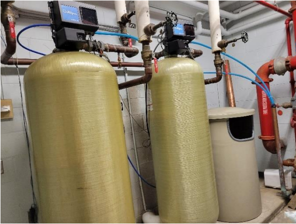
Photograph No. 41 Domestic cold water is treated with a softening system.
