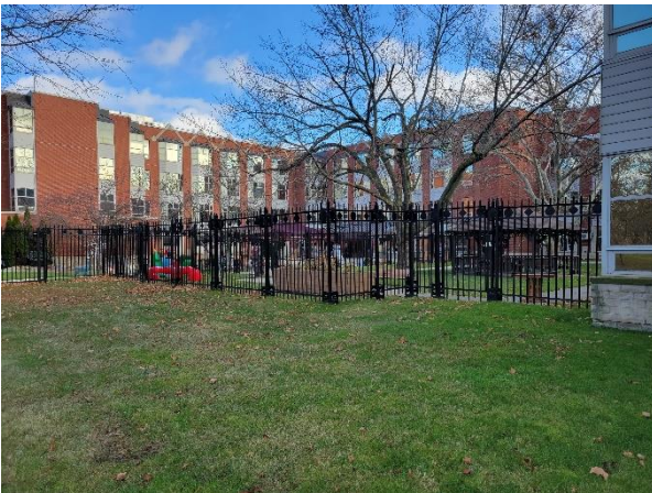
Photograph No. 67 Metal fencing around the rear outdoor area is in good condition.
