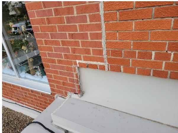
Photograph No. 12 Brick generally in good condition at south and main wings.
