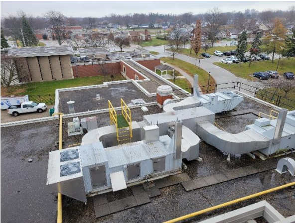
Photograph No. 15 Ponding water along south roof areas.
