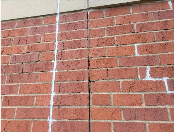
Photograph No. 9 Failed expansion joints at brick veneer.
