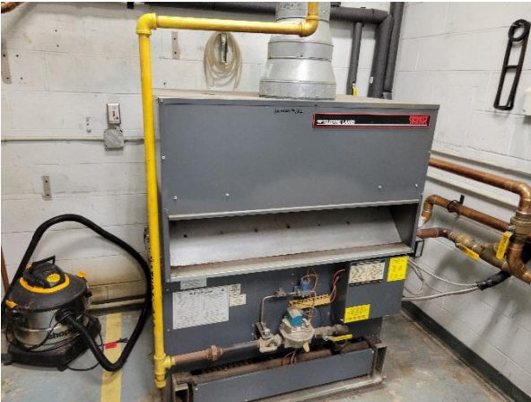
Photograph No. 59 Laundry boiler is older and will require replacement based on service life.
