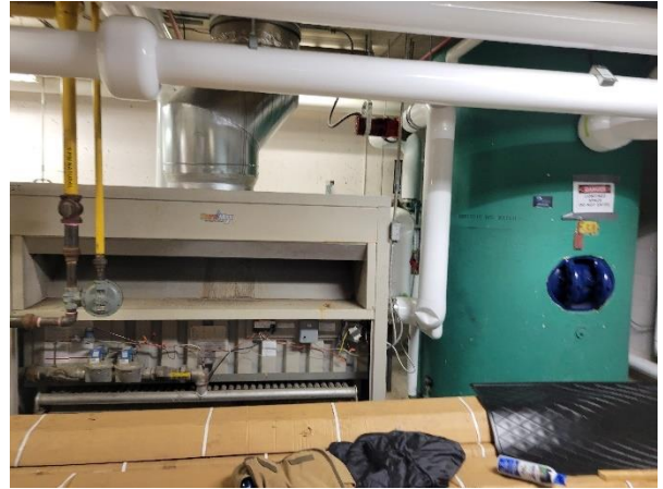
Photograph No. 42 Domestic hot water heater and storage tanks are operational with repairs recently completed.
