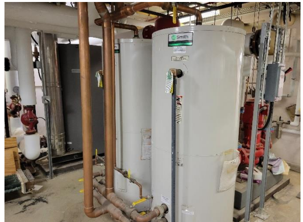
Photograph No. 44 Back-up DHW tank heaters are in good condition.
