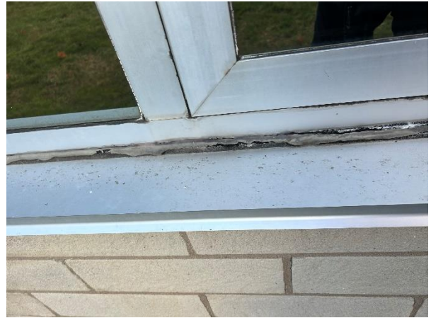
Photograph No. 6 Failed caulking at window perimeter.
