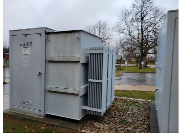
Photograph No. 50 Main power is supplied from pad mounted transformers.
