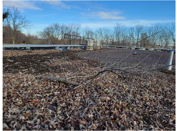
Photograph No. 18 Buildup of vegetation on garage roof.
