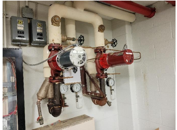
Photograph No. 60 Circulation pumps for the south wing heating loops appear to be operating normally.
