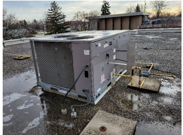
Photograph No. 52 South wing package rooftop units are in good condition.
