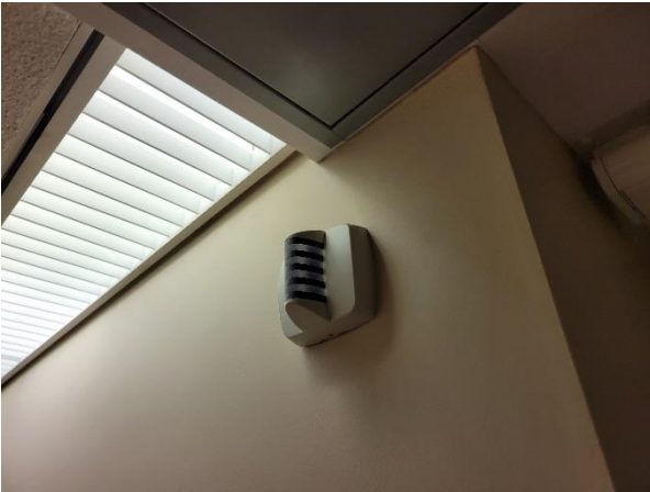
Photograph No. 55 Nurse call system is new and in good condition.
