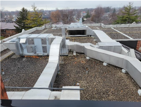
Photograph No. 47 All air handling units are in good condition.
