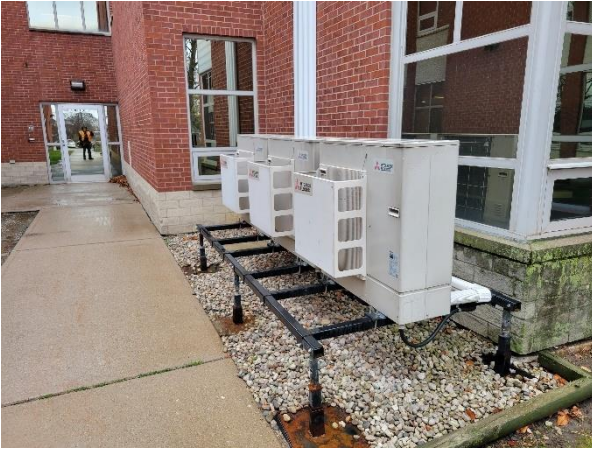
Photograph No. 49 Exterior condenser units are new and in good condition.
