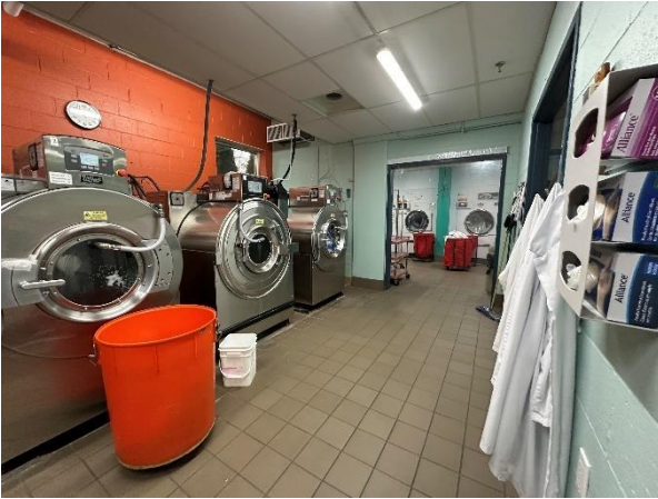
Photograph No. 33 Laundry room finishes, and equipment are in good condition.
