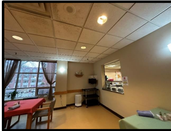
Photo 12: Typical lighting in common spaces.
