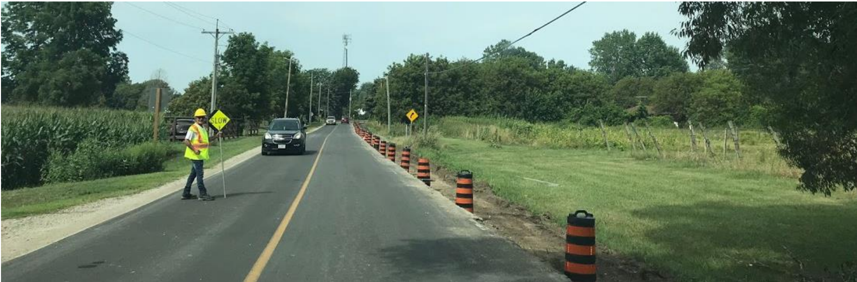
Figure 114: Road construction along County Road 50 in Oxley (implementation of paved shoulders along CWATS network) Source: WSP Canada
