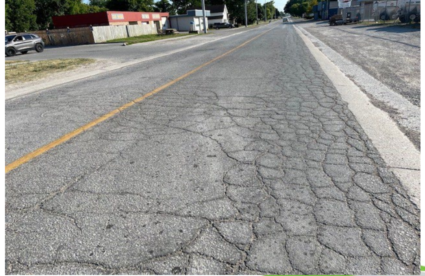
Poor to Very Poor Condition
