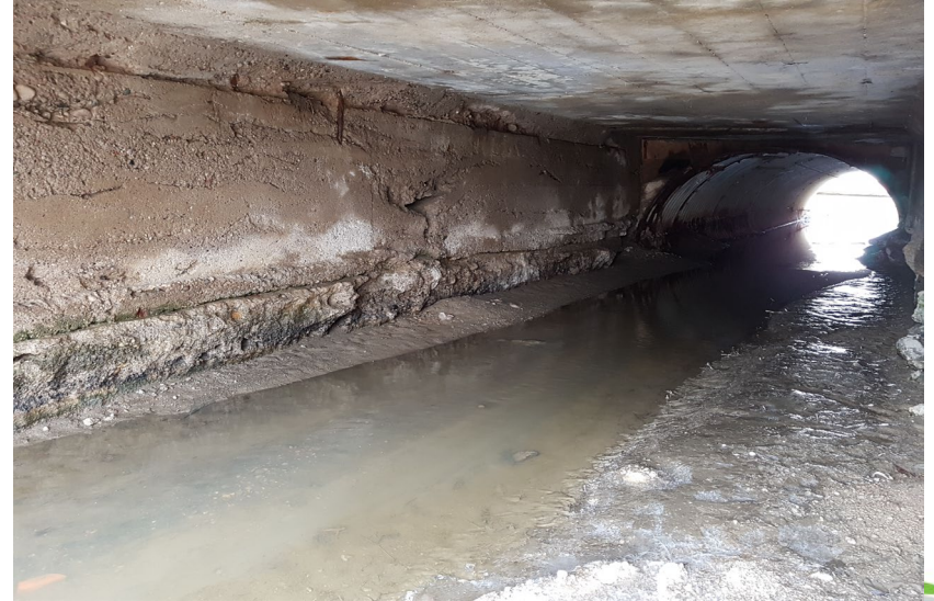
Poor to Very Poor Condition
