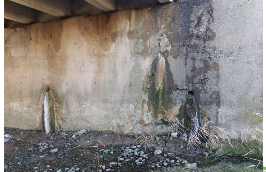
Poor to Very Poor Condition
